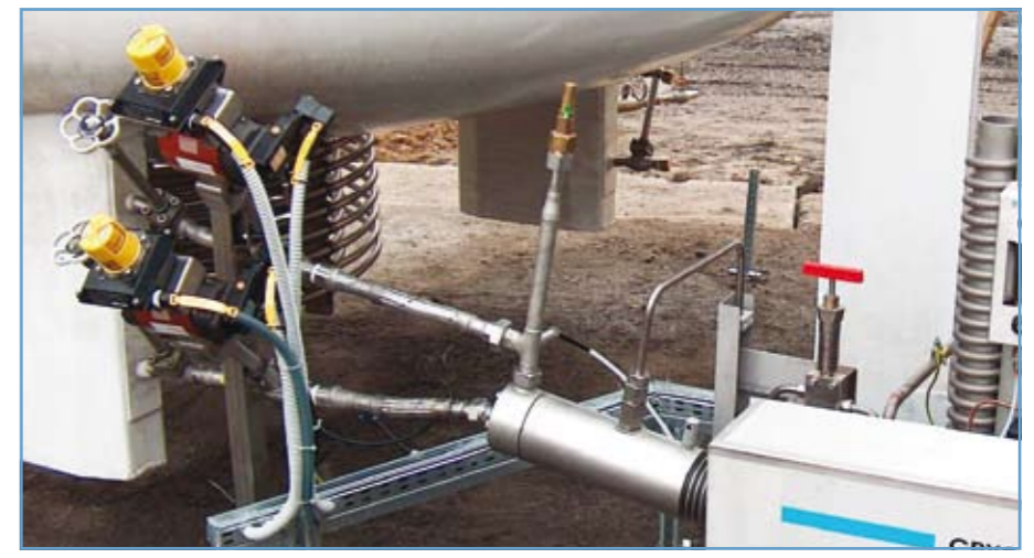
Typical thermosiphon installation with a high-pressure pump and actuated shut off valves
